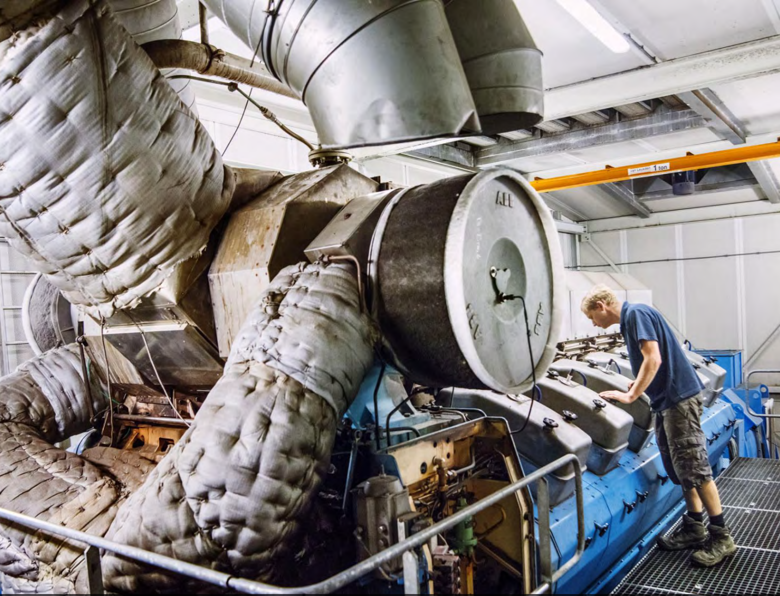
Tomato grower Jasper Oussoren checks a generator that converts natural gas into electricity for lighting. By-products—heat and CO 2 —are captured and used to warm greenhouses and boost plant growth.
